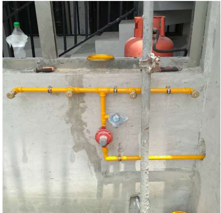
Gas line with Manifold and Gauge
