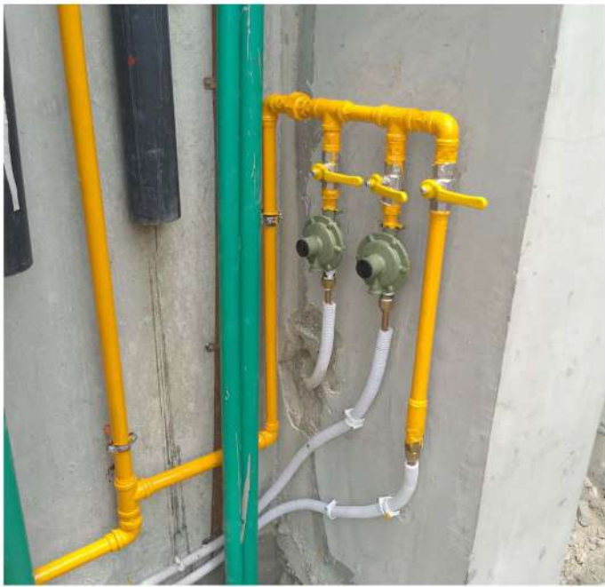
Gas manifold and Valve control
