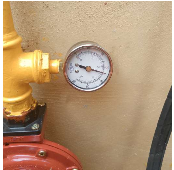
Manifold and Gauge Installation
