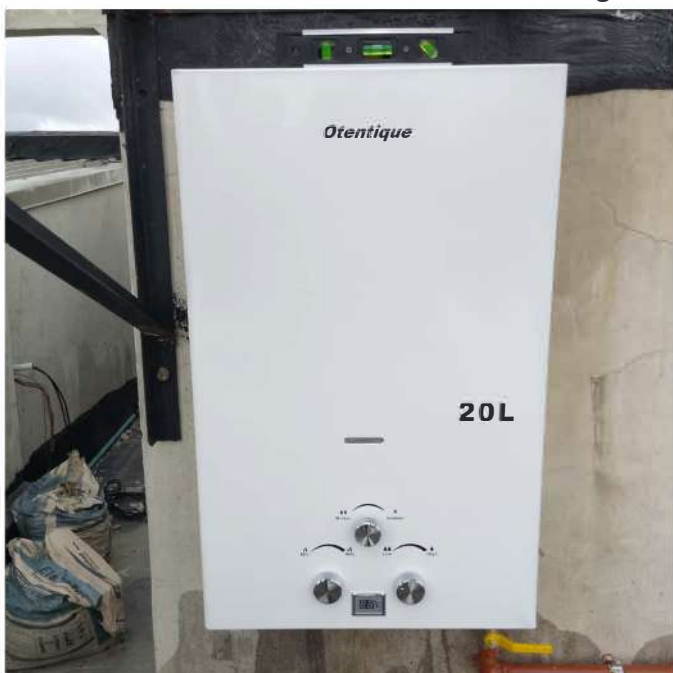
Installed Gas water heater
