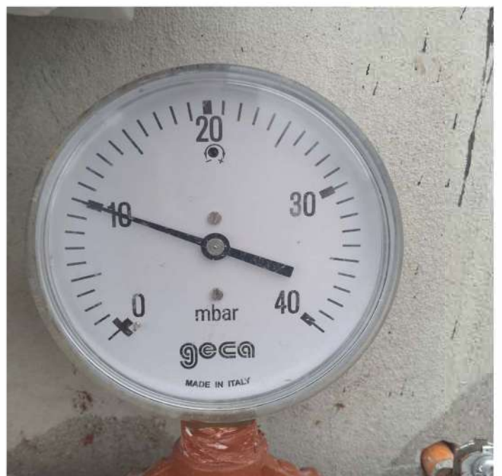
Gas Gauge with gas flowing
