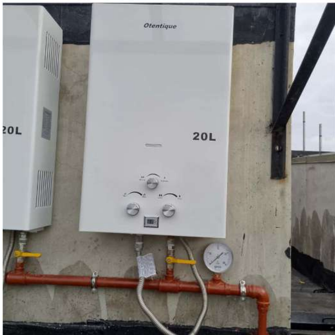
Gas water Heater with control valve and Gauge
