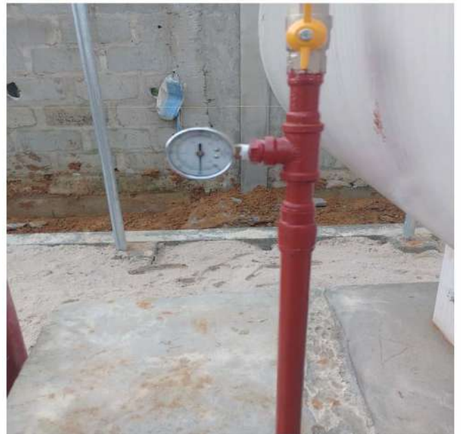
Gas Manifold with Pressure Gauge
