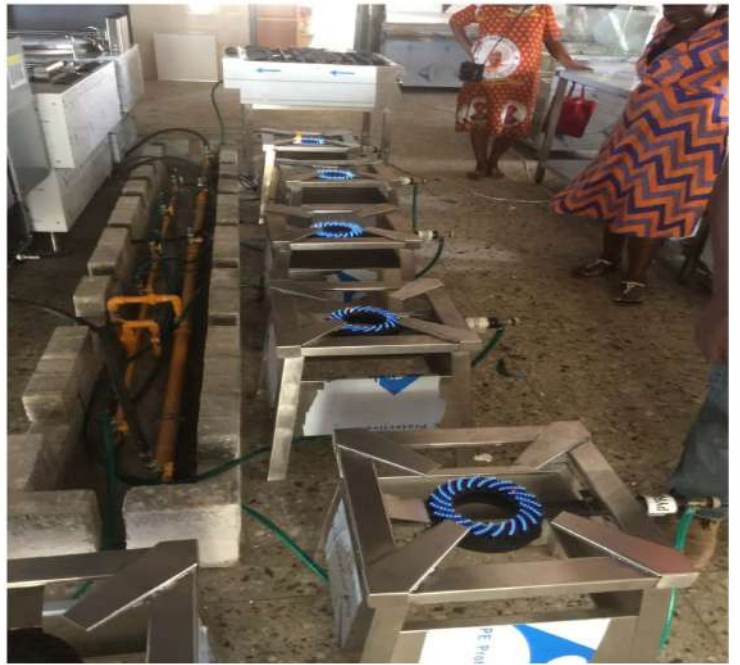
Installed Kitchen Equipment
