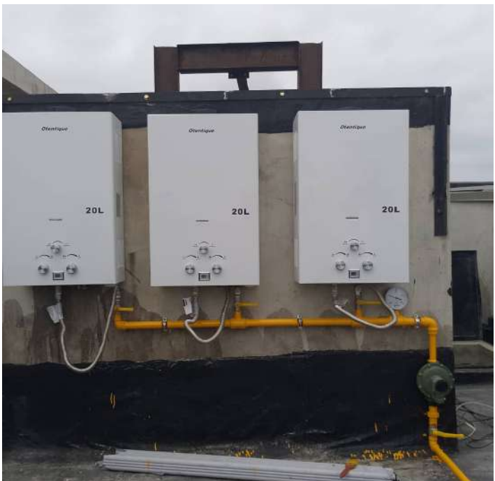
Intsalled Gas Water Heaters at Ikoyi, Lagos state.
