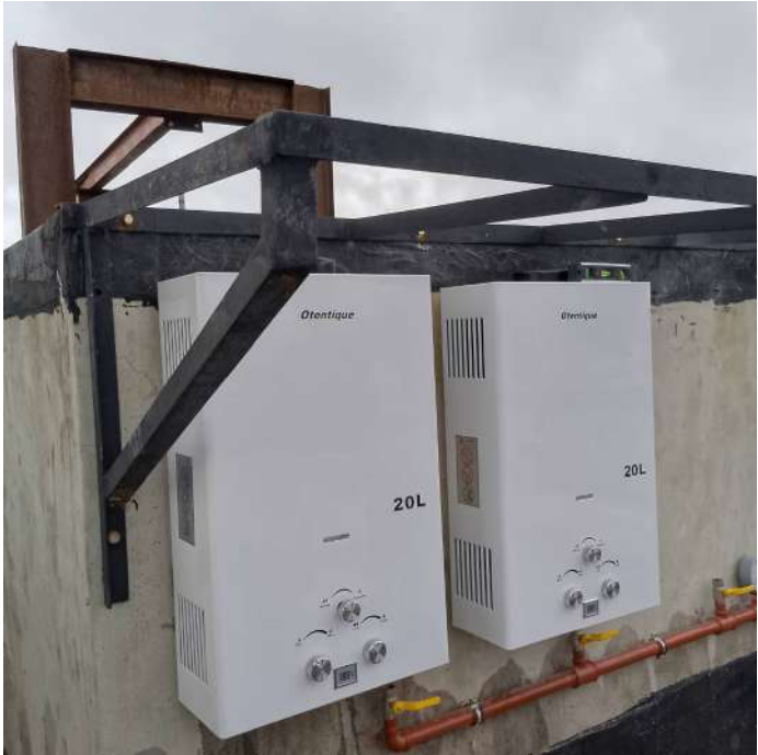
Intsalled Gas Water Heaters at Ikoyi, Lagos state
