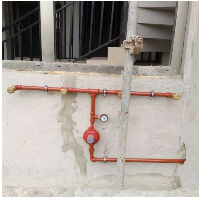
Gas line with Manifold and Gauge
