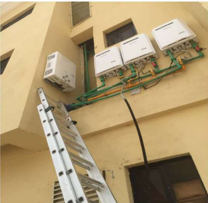
Installed Otentique Gas Water Heaters
